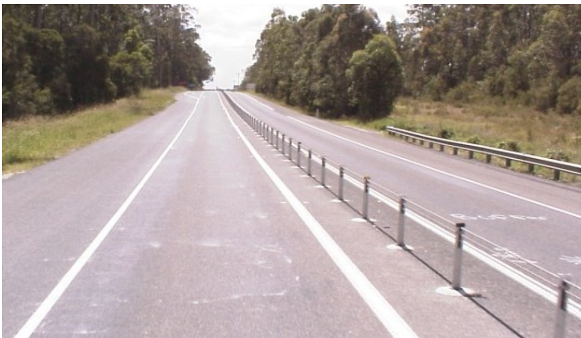
Image 5 - 2.0 metre wide Wire Rope Safety Barrier median – Pacific Hwy, at New Italy
