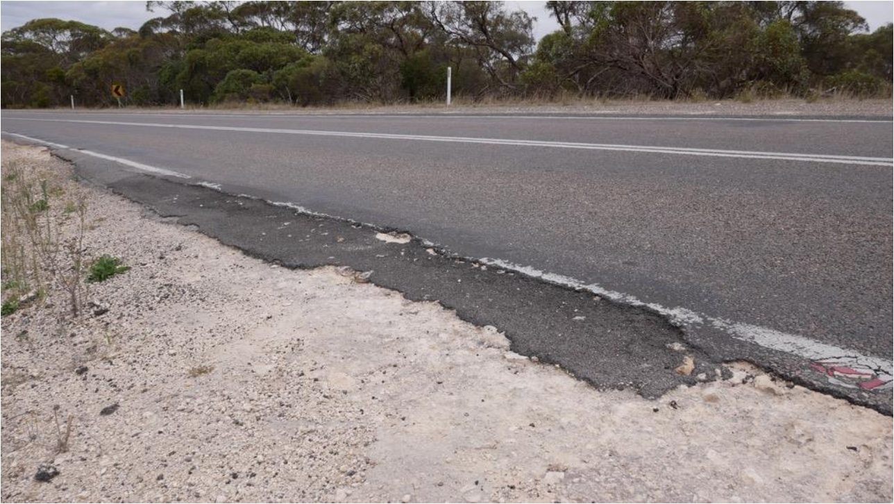
Figure 2.13 Example of a site photograph where the road edge has uneven remedial patching
